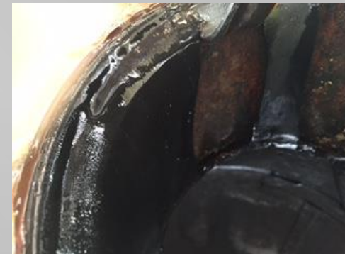
Crystallizer missing rubber liner
