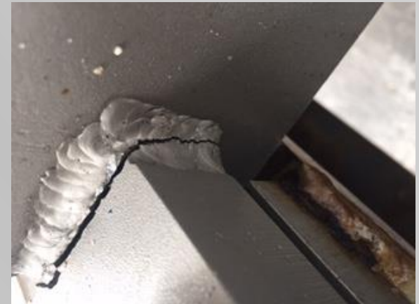
F. Press weld failure
