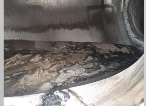
Door at mist eliminator
